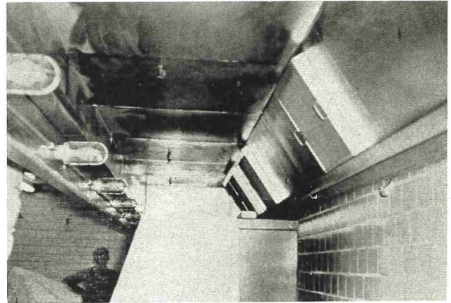
Figure 1. New ventilation hood with easily removable grease filters, adequate easily removable light fixtures, and easily cleanable walls behind permanent equipment.
